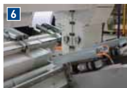
6 Wireless Rewind Arm Positioning Rewind arms are positioned using industrial 'Bluetooth' technology which also sends speed and tension references automatically to the drives. Power is provided by a DC bus bar located under the rewind beams.
